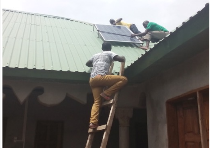
Solar electricity has been installed in the guesthouse
