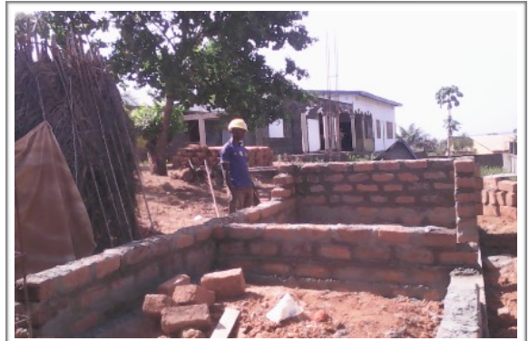
A small office and store room has been started for the water project and it's materials
